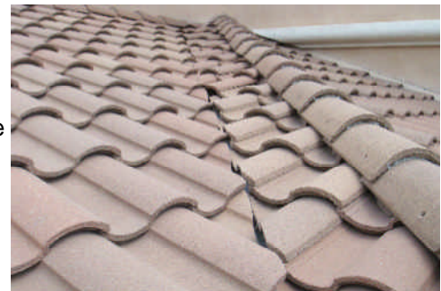
Closed valley may restrict water runoff.
