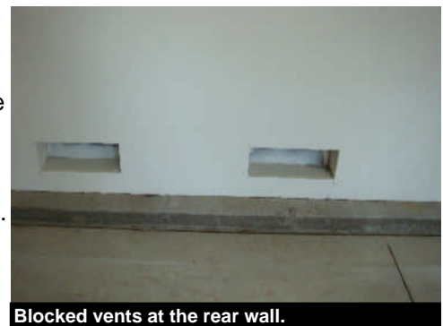
Blocked vents at the rear wall.
