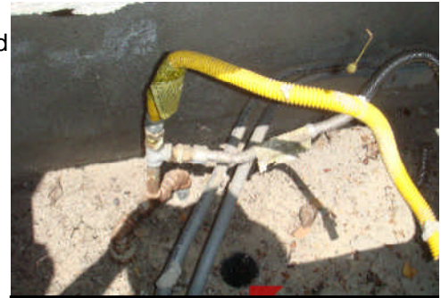
Surface drain is lacking cover.
