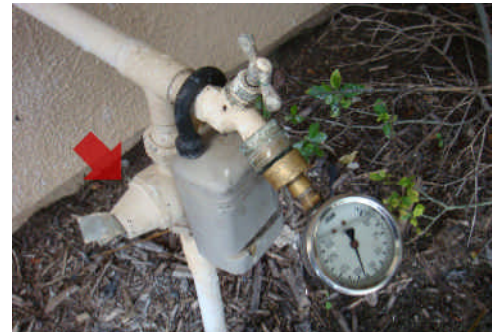
Excessive water pressure. Replace Reg.
