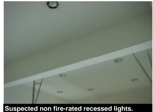
Suspected non fire-rated recessed lights.
