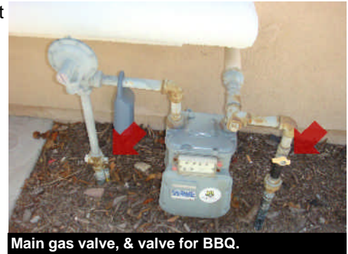
Main gas valve, & valve for BBQ.
