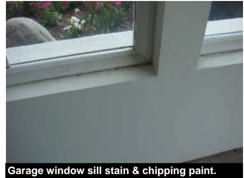
Garage window sill stain & chipping paint.
