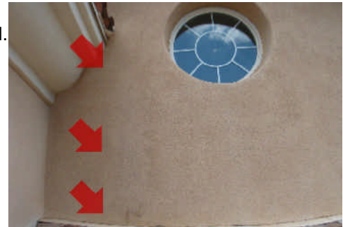
Discolored stucco below roof flashing.
