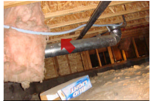
Unsecured wiring & insulation below kit.
