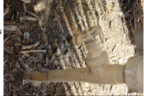
View of the original main water valve.
