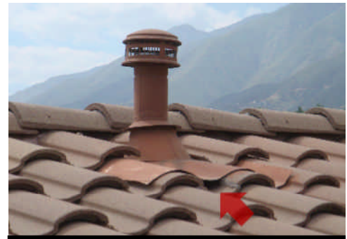
Void /opening below flashing.
