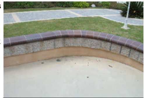
Front walls are lacking guard railings.
