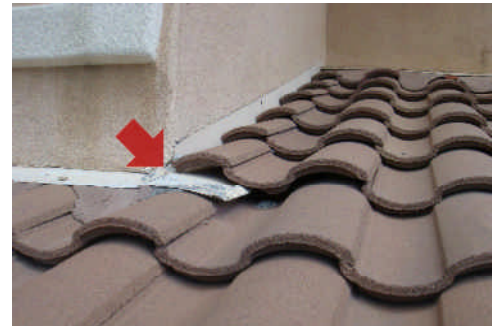
Lifted pan flashing & void at the front.
