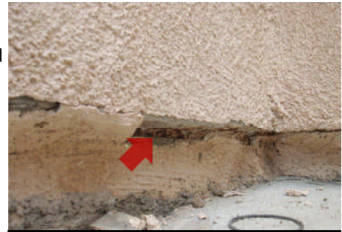
The stucco screed is rusting.
