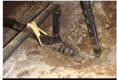
View of the main drain line at rear left.
