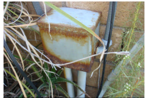
Rear rusted junction box.
